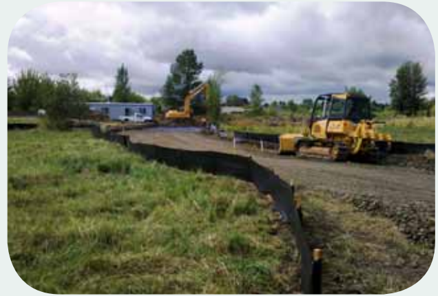
Ground preparation began in July on the hospice house site. Alton E. Sullivan Construction is preparing the foundation for the facility. T. Gerding is the general contractor with Dan Bates serving as T. Gerding’s project superintendent.
