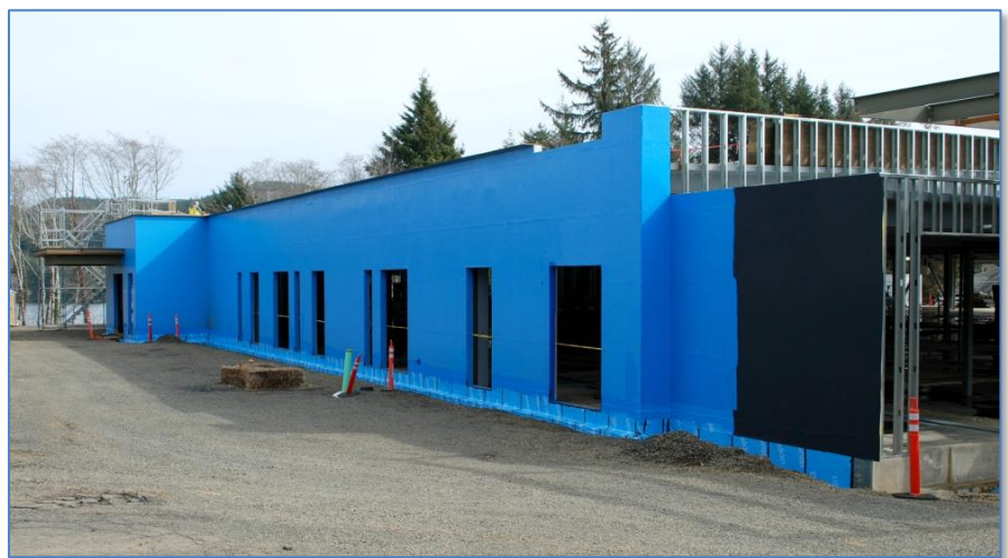
Top photo shows southwest corner of the new building, and bottom photo shows west side of the building (helipad is out just steps away).
